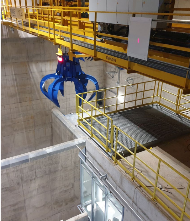
Fuel bunker with waste grab shown prior to waste deliveries
