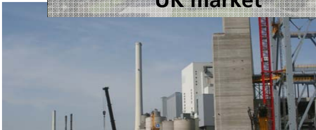
Expansion in district heating Block 9 GKM
