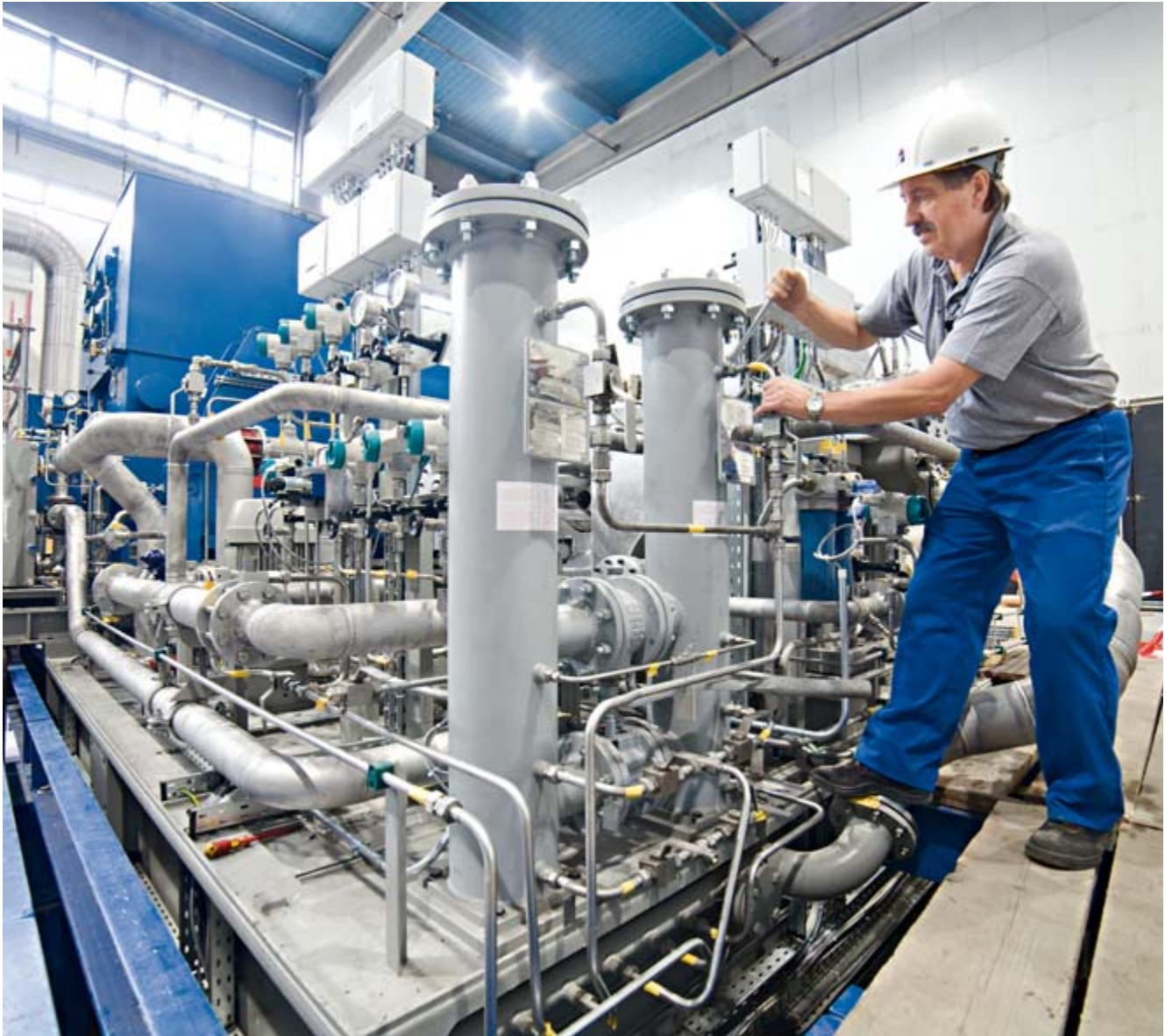
• One of the two back-pressure steam turbines in the OptiMa project (here Turbine D0) shortly before trial operations
