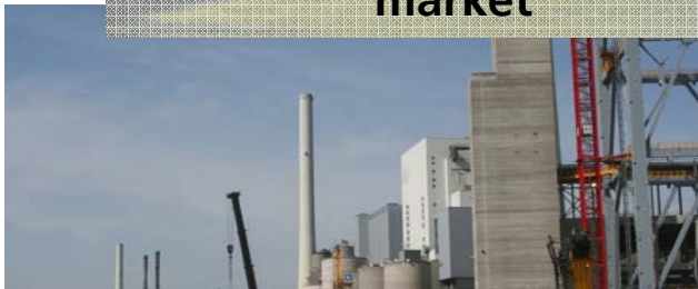
Expansion in district heating Block 9 GKM
